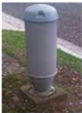
Recognise this? It is the node in fibre to the node connections. Image courtesy of Department of Communications.
